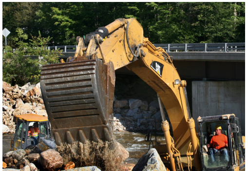
Debris had to be cleared in many rivers and streams throughout Vermont as a result of flooding from tropical storm Irene. FEMA News Photo.
